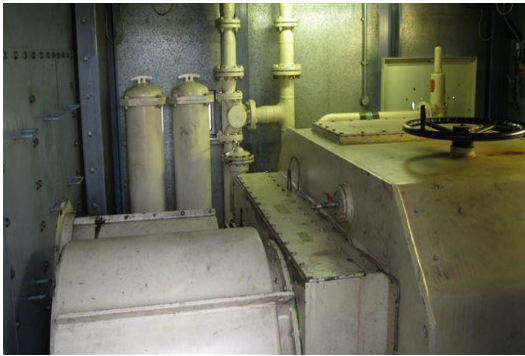
Lube oil generator/gearbox
