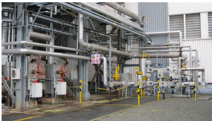
Natural gas reduction station and steam heating NG
